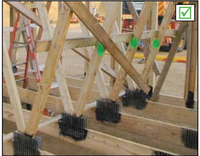
Install Web Member Permanent Lateral Restraint and Diagonal Bracing (or web reinforcement) and Bottom Chord Permanent Lateral Restraint and Diagonal Bracing as required.
