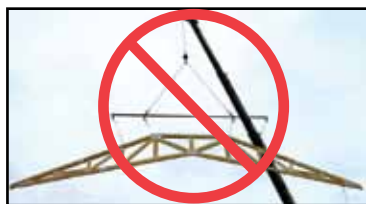
Spreader Bar used is too short for this Truss.
