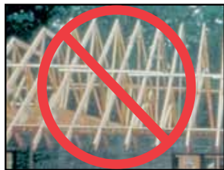
Improper bracing scheme - Continuous TCTLR without Diagonal Bracing
